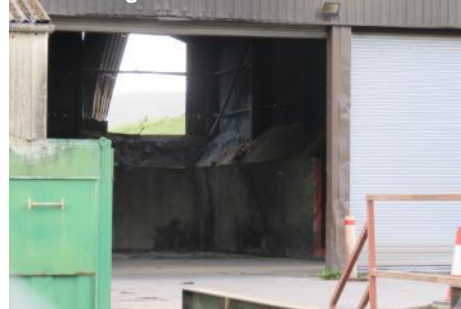
Fire damage to the waste transfer station
