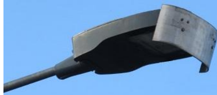
While most are pleased with their new street lights, a few find them a hindrance. It's possible to place a 'shield' on an LED to concentrate their light downwards still further, as seen on this lantern on Denbigh Road
