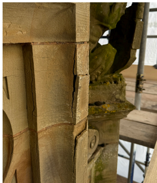
Holli haenau cyn cyflawni'r gwaith adfer Delaminating/splitting of layers before restoration
