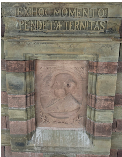
Tystiolaeth o lanhau cemegol gydag asidau a arweiniodd at losgiadau a staenio Evidence of chemical cleaning with acids resulting in staining and burns
