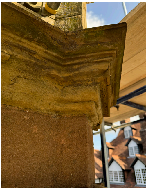
Cyflwr y cornis diffygiol cyn y gwaith adfer Condition of the defective cornice before restoration work
